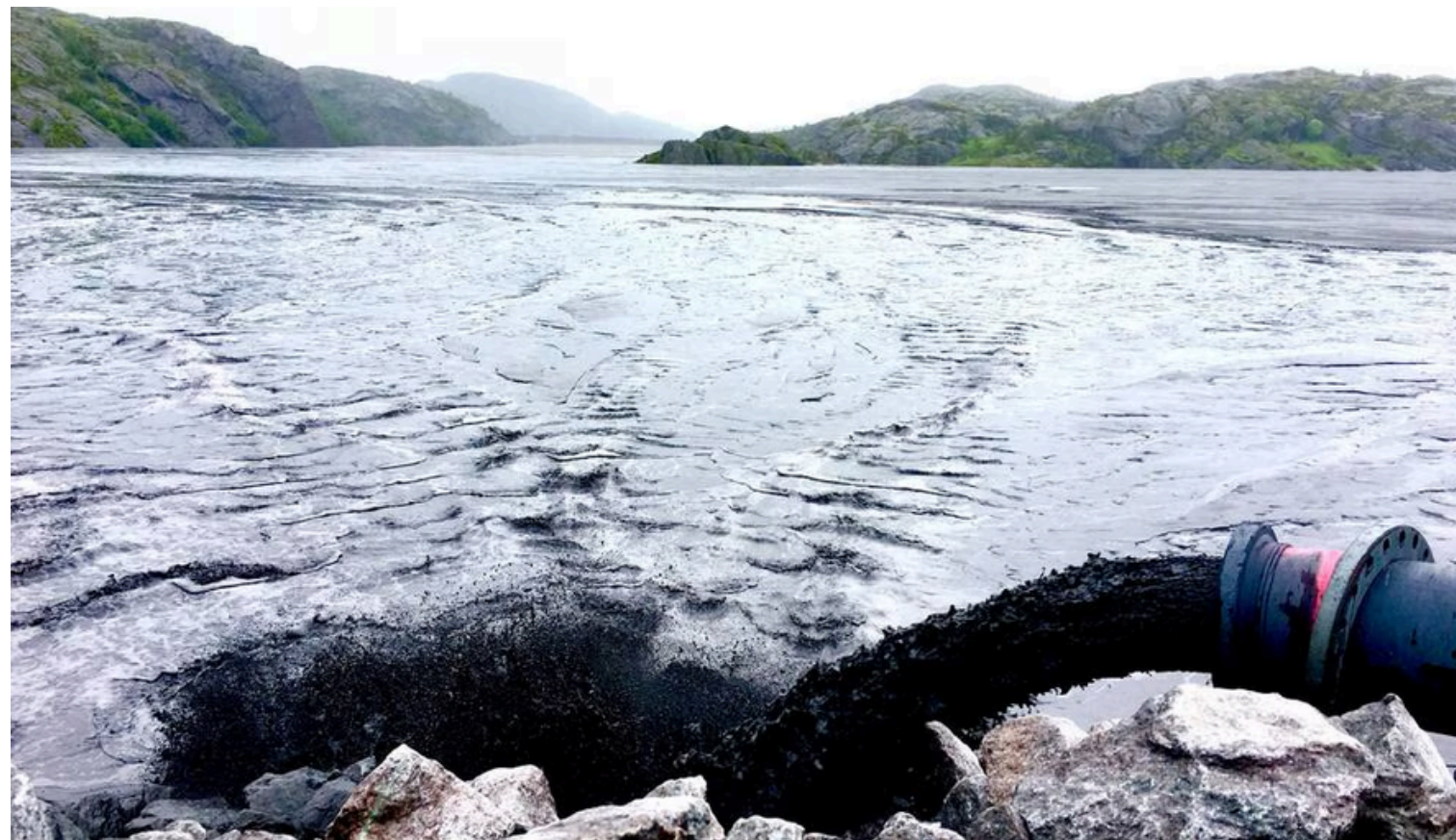
TSF land fill from the Titania mine in Sokndal, Norway. Without watering, dry tailings from the Titania TSF would create significant dust pollution. It's necessary to mitigate this substantial water application performed through manual watering using tractors and sprinkler systems. Photo: Mathias Oppedal.
