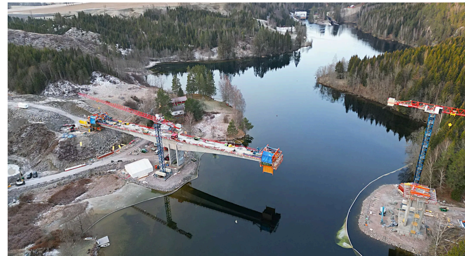
The new bridge along fylkesvei 359 is under construction and is set to open later in 2025. Photo: Olav Heggernes/Telemark Fk
