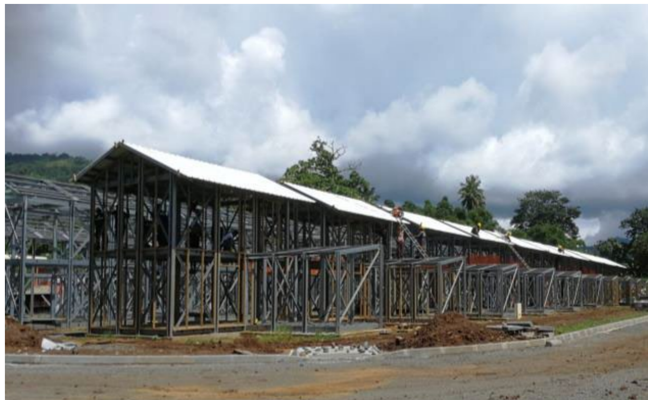
THE VILLAGE-RELAY ÉTAPE FULERA: ASSEMBLY OF METAL STRUCTURES (TOP) AND COMPLETION OF THE SITE (BOTTOM) EPFAM, 2022
