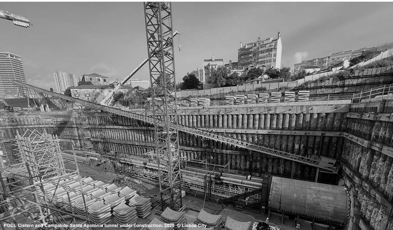
PGDL Cistern and starting the construction of the Campolide-Santa Apolónia tunnel © Lisboa City
